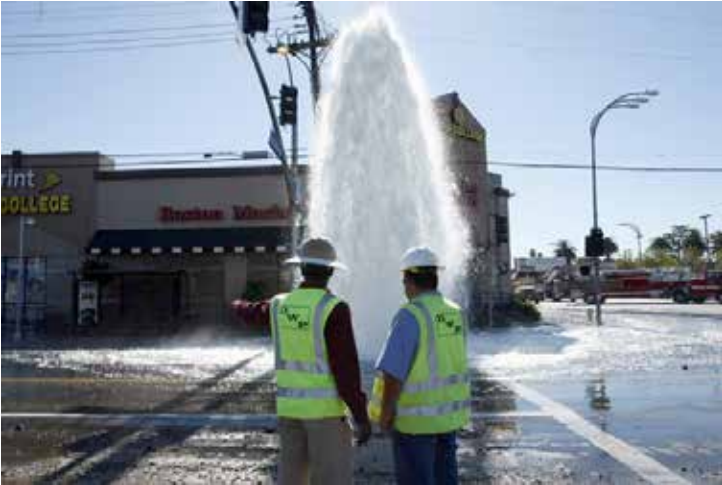
Syracuse saw a record 372 water main breaks in 2015 due to aging pipes and a lack of funds to repair them.
